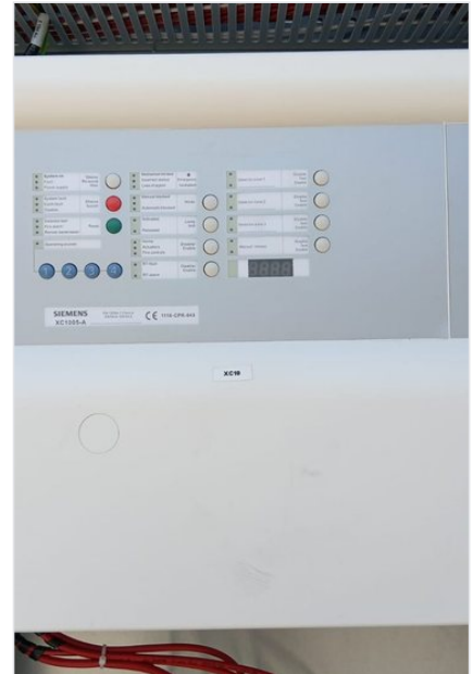
Siemens XC1005-A extinguishing panel
