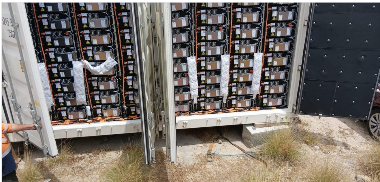
Both battery bays open, all module strings in situ
