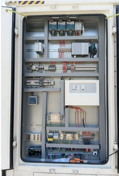
Auxiliary control cabinet
