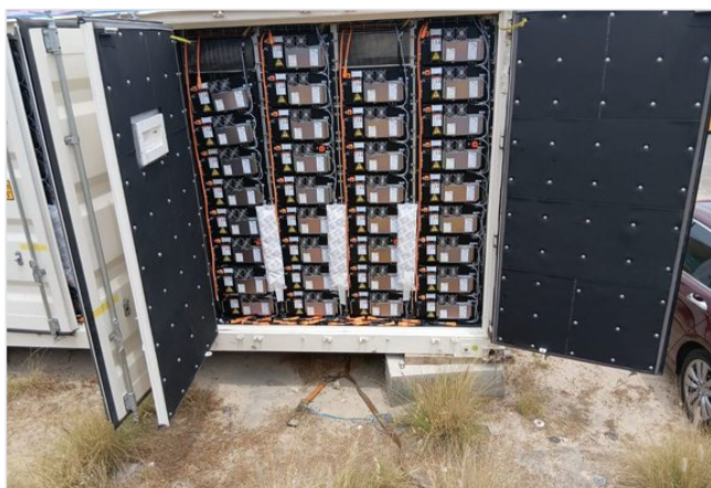
Single bay detail, racks and harnessing intact
