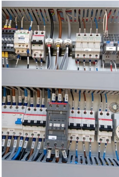
Distribution, contactors and protection
