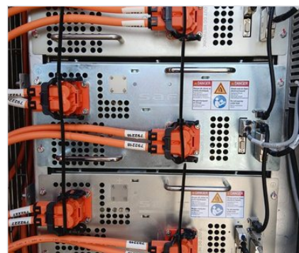
Saft modules with SMUs as installed
