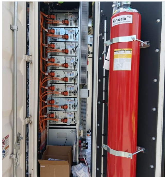
Battery room door open, Sinorix cylinder door mounted
